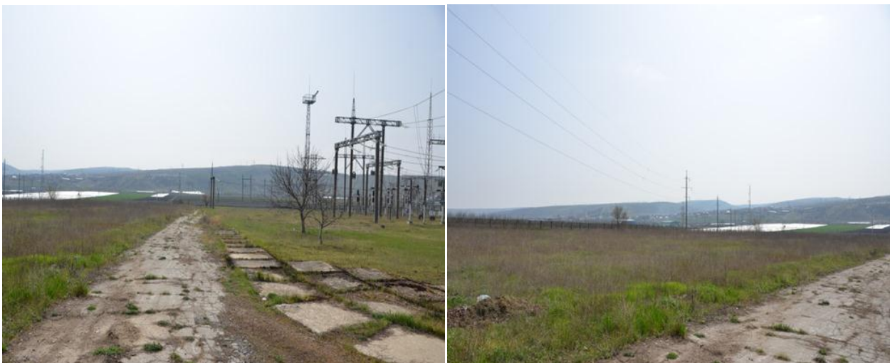
Figure 3.1.1.3 Free space inside 330/110/35 kV Chişinău station
