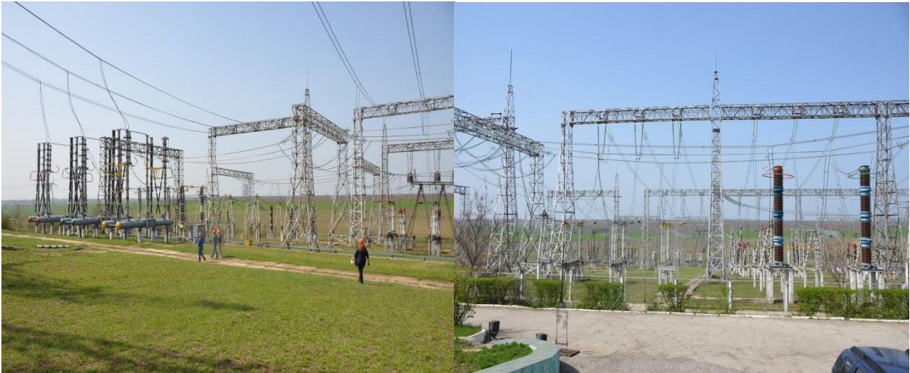
Figure 3.1.1.1 400/110/35 kV Vulcănești station
