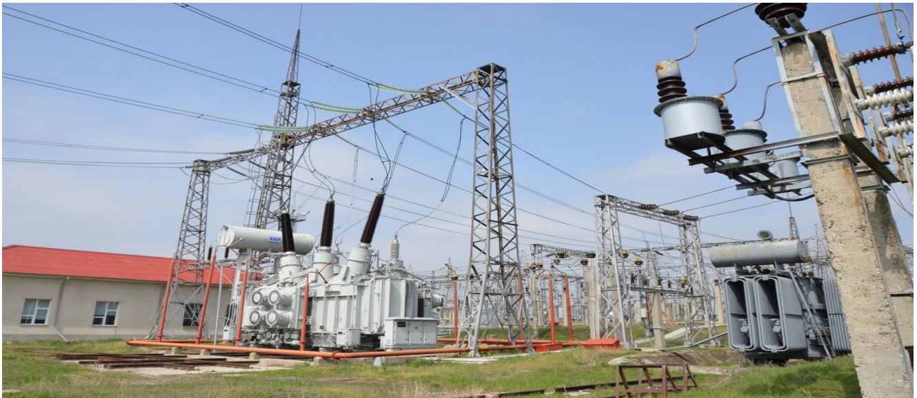
Figure 3.1.2.1 330/110/35 kV Chişinău station
